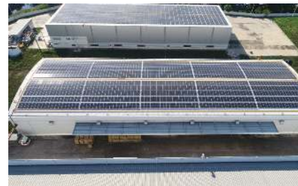
Sun Panels Installed at the NISSIN FOODS (THAILAND) Plant
