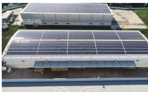
Solar Panels Installed at the NISSIN FOODS (THAILAND) CO., LTD. Plant
